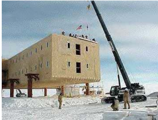
South Pole Rebuild - Independent structural and cold-regions engineering peer review performed by Gregersen Structural Engineering, Incorporated, Park City, Utah. (Photo courtesy of Raytheon Polar Services and The Arctic Sun)
